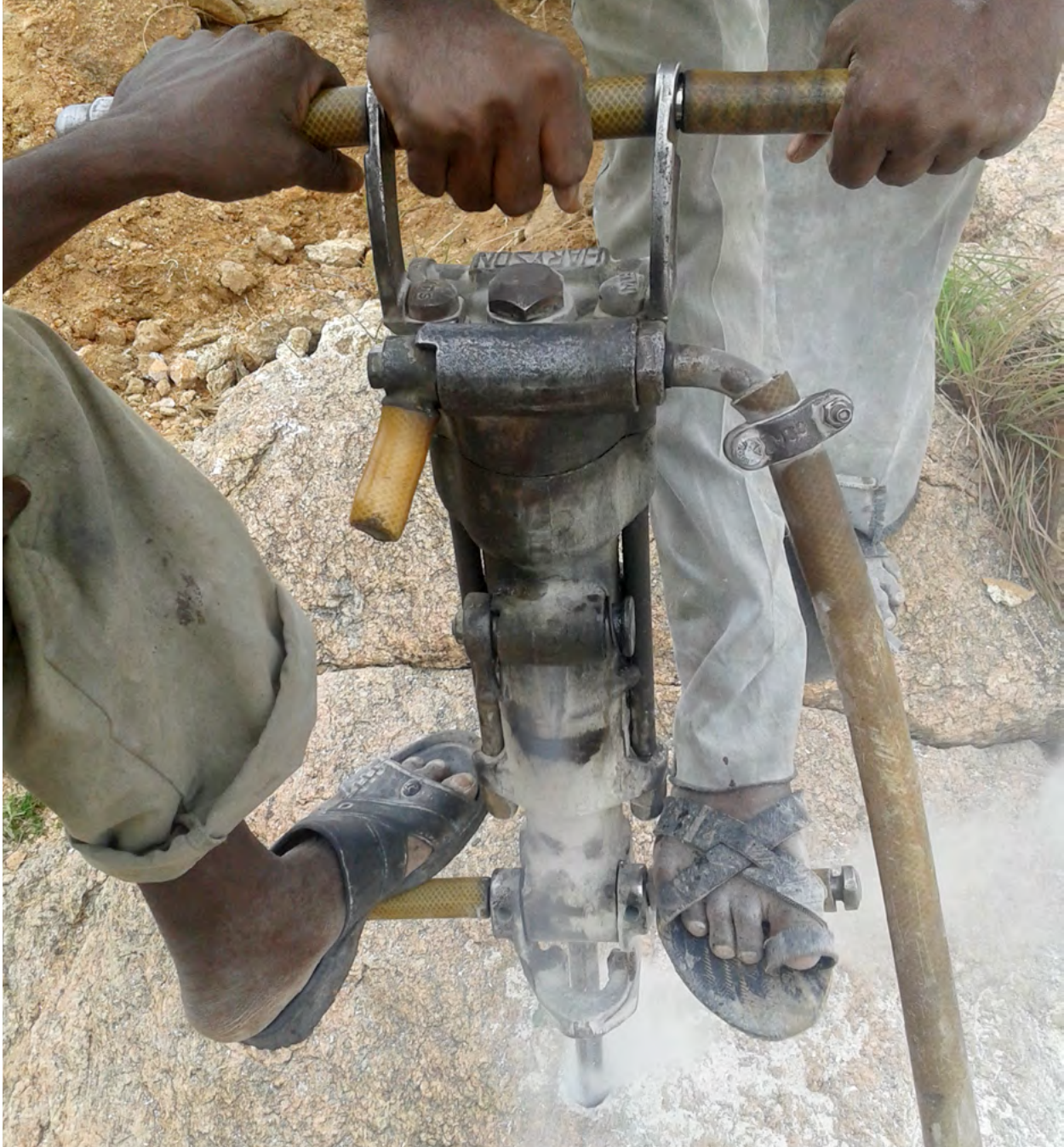
Quarry workers operating the drilling machine without using protective equipment
